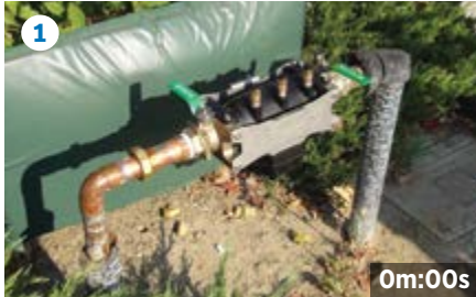
Backflow is installed with ball valves in the closed position.
