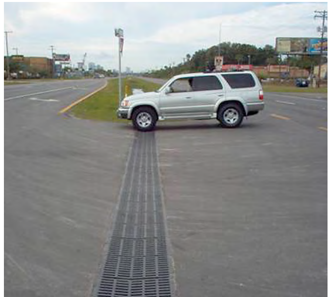
Highway - Z874-FL DOT Grate
